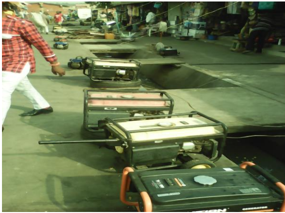
Plate II. Indiscriminate use of electricity generators to power appliances for artificial cooling and ventilation in Wuse Market. (Source: Researcher's field work, 2018).
